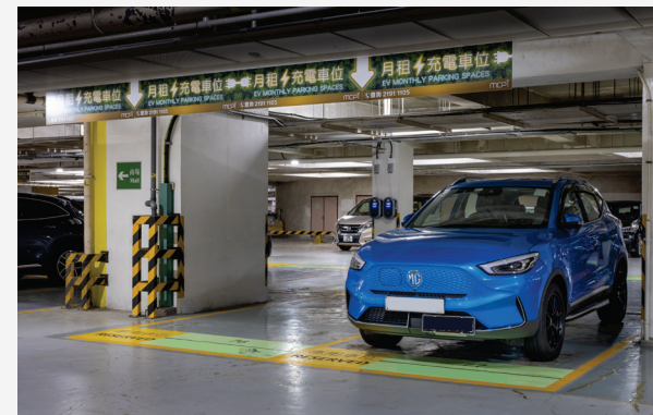
EV charging facilities at MCPI
